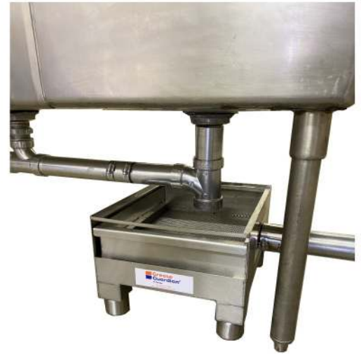
DS-1 solids filter installed under a 3 compartment sink.
